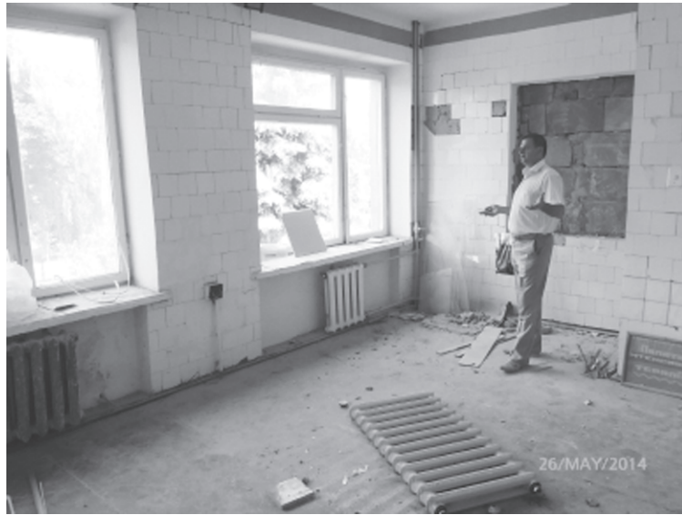
Volodya Polevay, MMC Raiyon manager. Tovsteh Care and Rehabilitation Centre in a third-floor room being renovated for disabled children.
